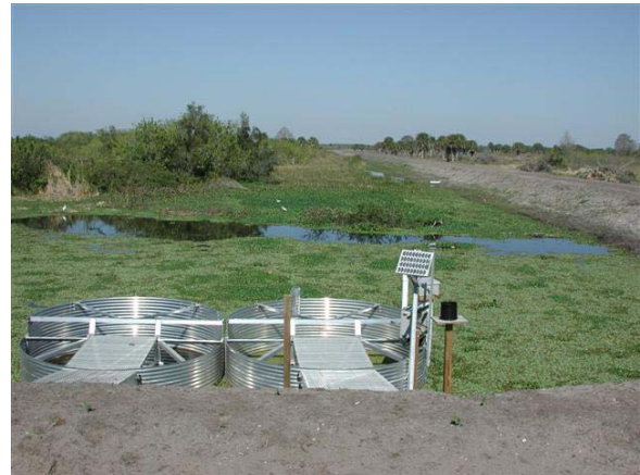
Outflow structure and water monitoring equipment installed on the Queen Bee Farms' wetland restoration project.
